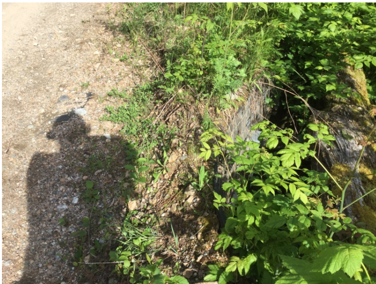
Downstream fill retention facing exposed to grader activity
