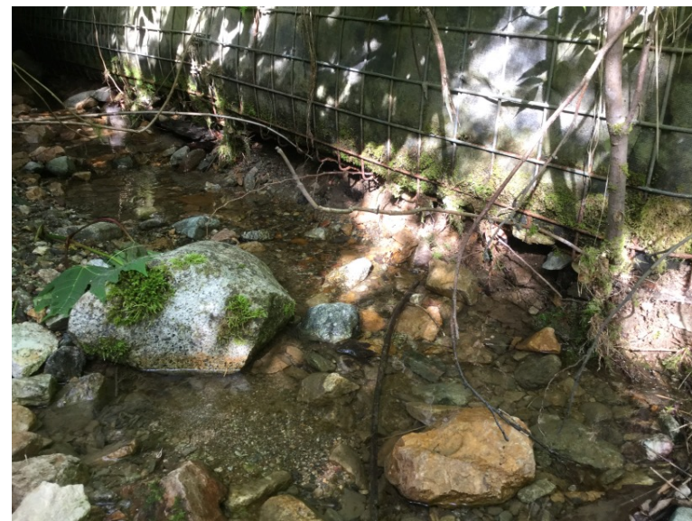
Foundation scour under downstream left bank abutment
